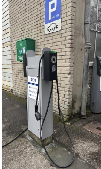
Figure 8 EV Charging stations installed in Massagno, Switzerland
